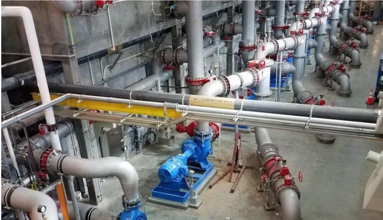
MID Water Treatment Facility
