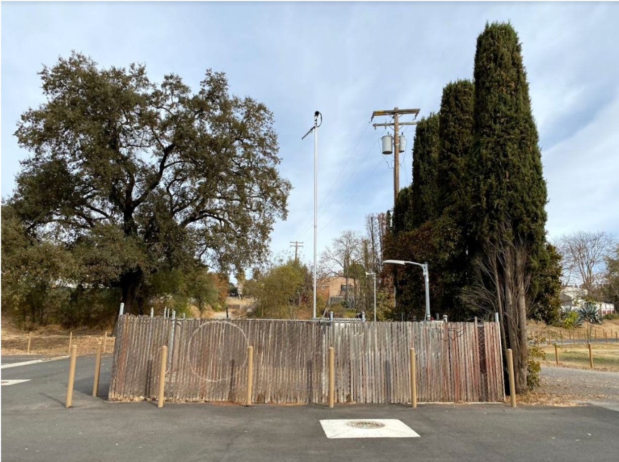
Photo 19. Waterford River Park - Lift Station
