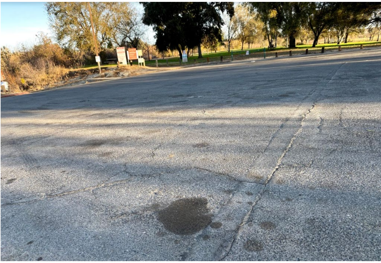
Photo 12. Fox Grove Park - oil stains all over in the parking lot
