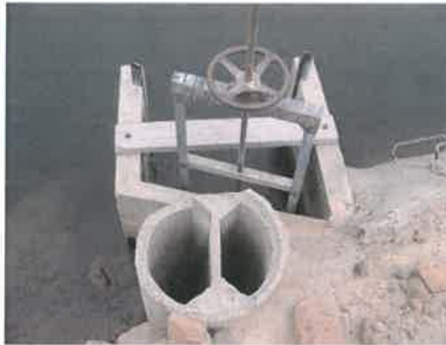
Figure B-9. An old type of dual-stilling well commonly found in Central California irrigation districts. One stilling well was connected to the canal, and the second was directly over the discharge pipe. The idea of measuring down into both stilling wells from the same center point was good, but the top of the stilling well was so close to the ground surface that road maintenance quickly filled these stilling wells with dirt. Also, the side connection between the canal stilling well and the canal itself was too difficult to clean.
