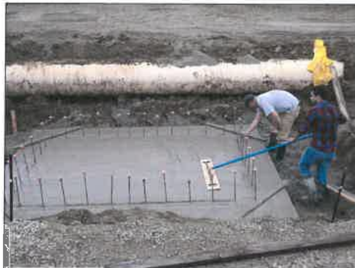
Figure A-3. Initial construction of main spill box that the meter gate pipeline drains into.
