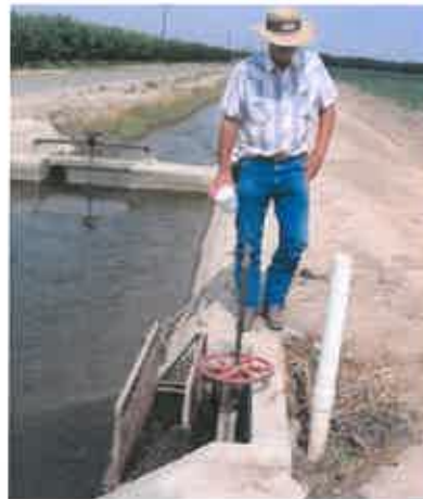
Figure B-10. This stilling well is properly located, but it has too small a diameter. The operator also needs to know the elevation difference between the top of the stilling well and the gate frame, which requires an extra computation to determine the difference in head across the gate.
