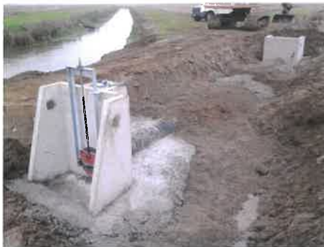
Figure B-16. Final concrete for GCID meter gate, showing downstream pre-cast outlet box.
