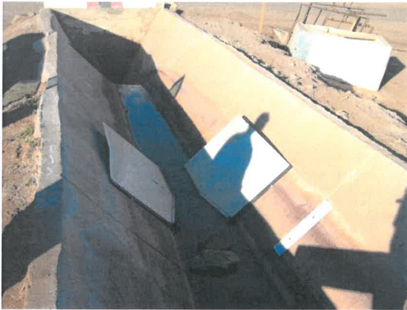
Figure 3. Side contractions rather than a traditional "Replogle Flume". Designed by USBR, Yuma. The rocks are not part of the design.
