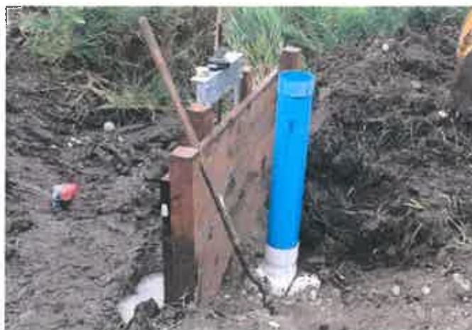
Figure B-8. Stilling well installed on an existing discharge pipe. It is constructed of PVC pipe that is too thin for long life, but it serves as an example of the correct diameter, position, and height.
