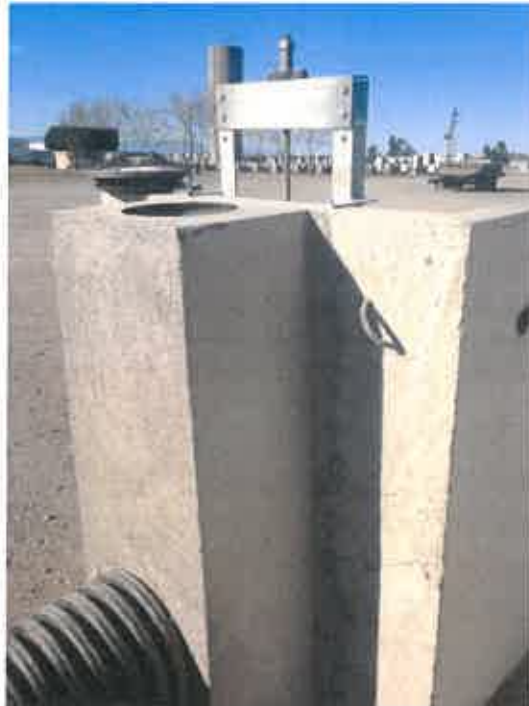
Figure B-13. GCID meter gate at Briggs
