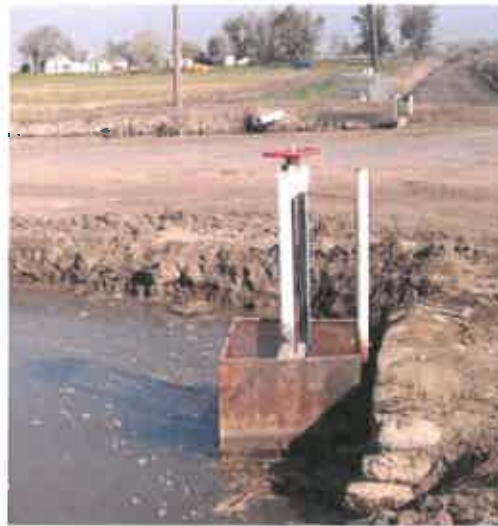
Figure B-11. Correct height of stilling well to match top of gate frame. However, the diameter is too small. Steel pipe material is good
