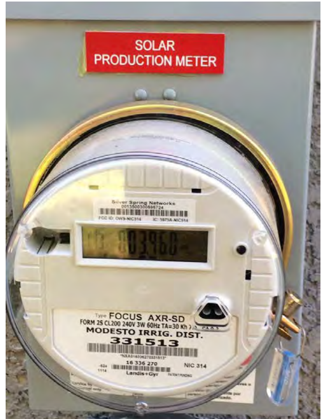
Figure 4: Solar Production Placard
