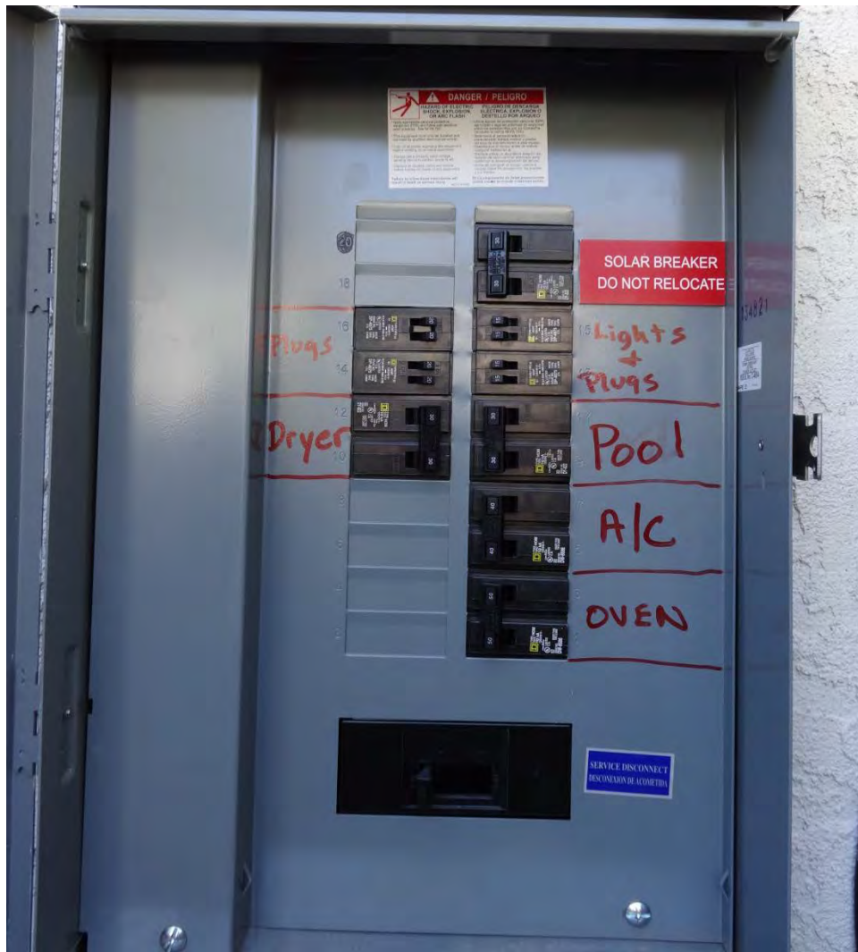
Figure 5: Solar Breaker Placard
