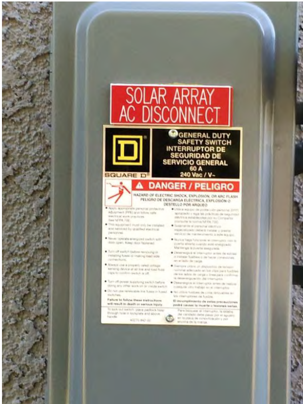
Figure 2: Solar Array AC Disconnect Placard
