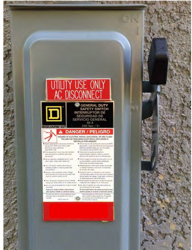
Figure 3: Utility Use Only AC Disconnect Placard
